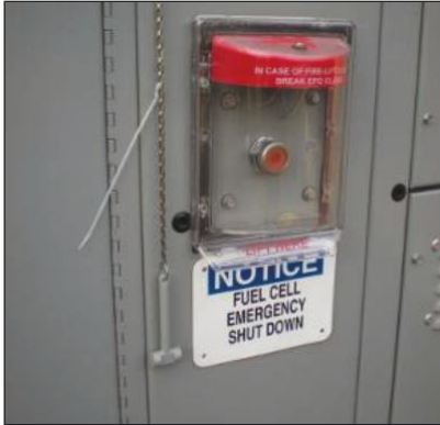
Figure 1: Emergency Power Off Button
