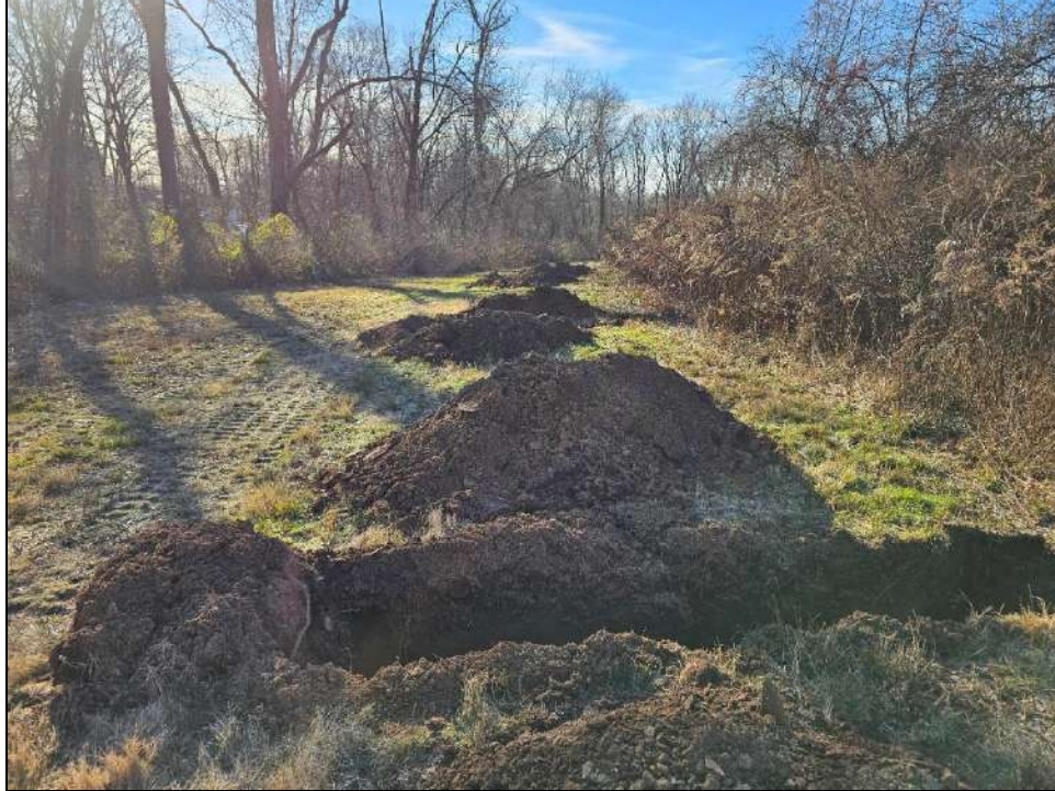
Photo 3. Previously excavated trenches identified along the eastern boundary of the Northern Field. Photo taken facing south.
