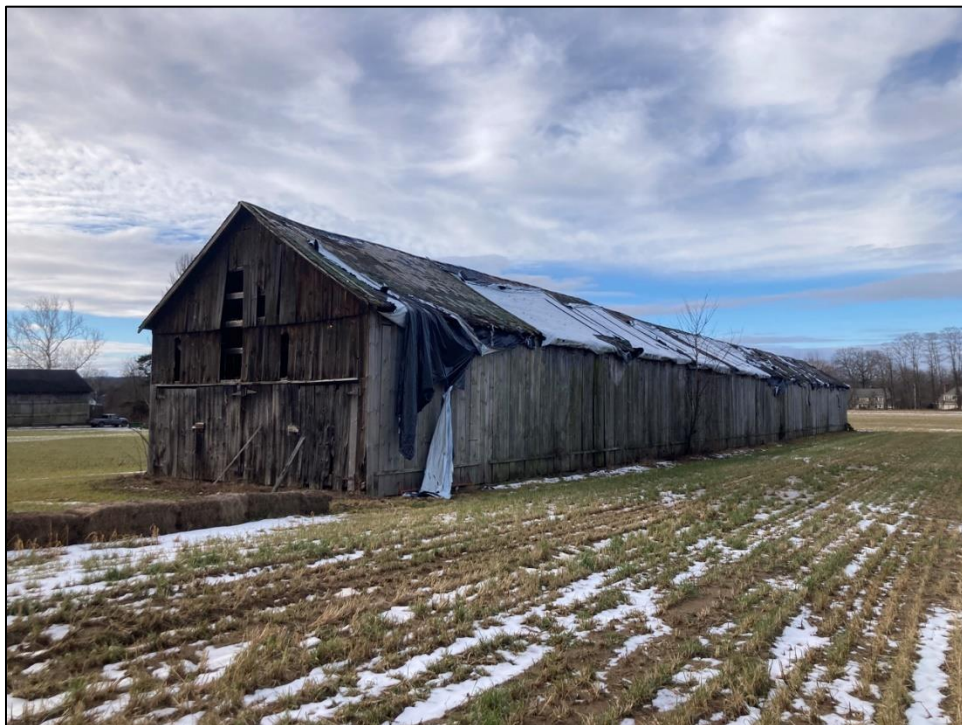
Photo 16. 3/4 view of the east elevation of Structure 2. Photo facing to the southwest.
