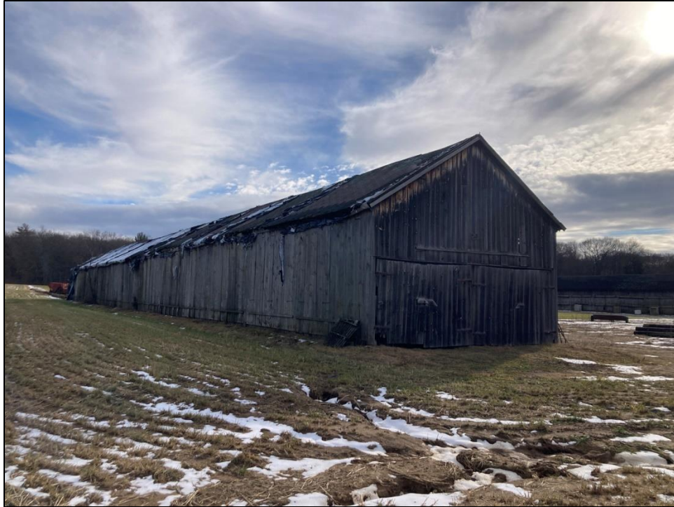
Photo 15. 3/4 view of the west elevation of Structure 2. Photo facing to the southeast.
