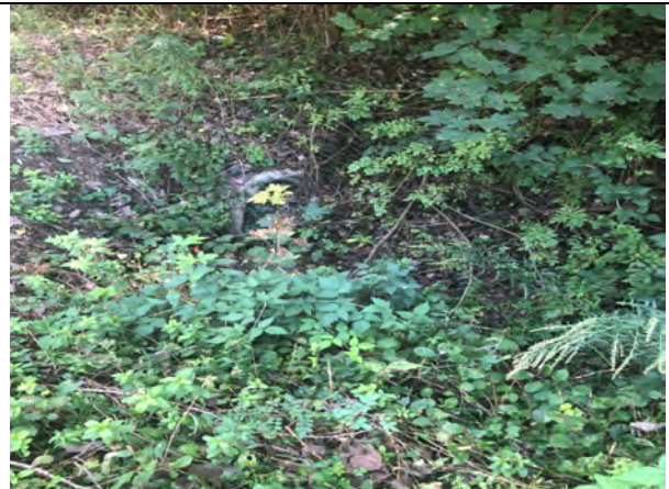
Photo 18: Discharge culvert pipe for landfill drainage swales.
