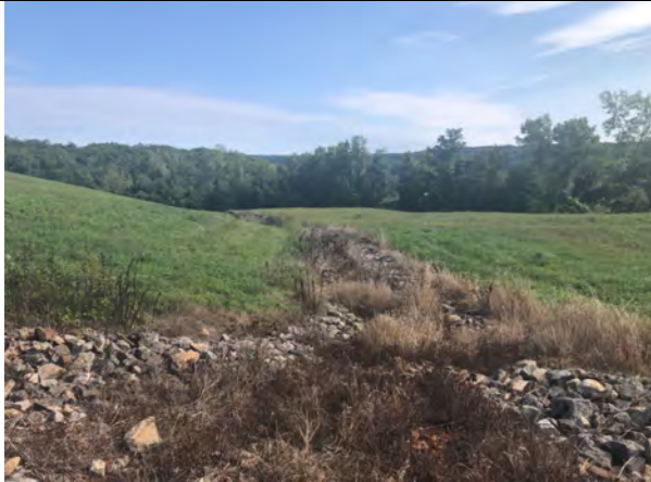
Photo 9: Looking northeast along drainage swale east side of municipal waste fill Area.
