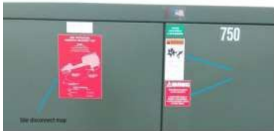
Typical Transformer Signage/ NFPA
