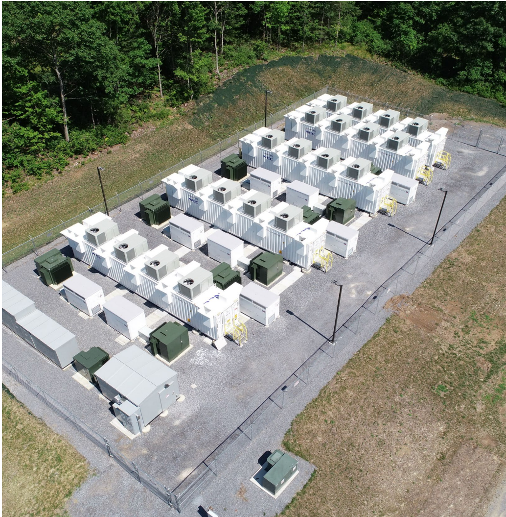
KCE's first operational project in New York, KCE NY 1, 20 MW/14.4 MWh BESS
