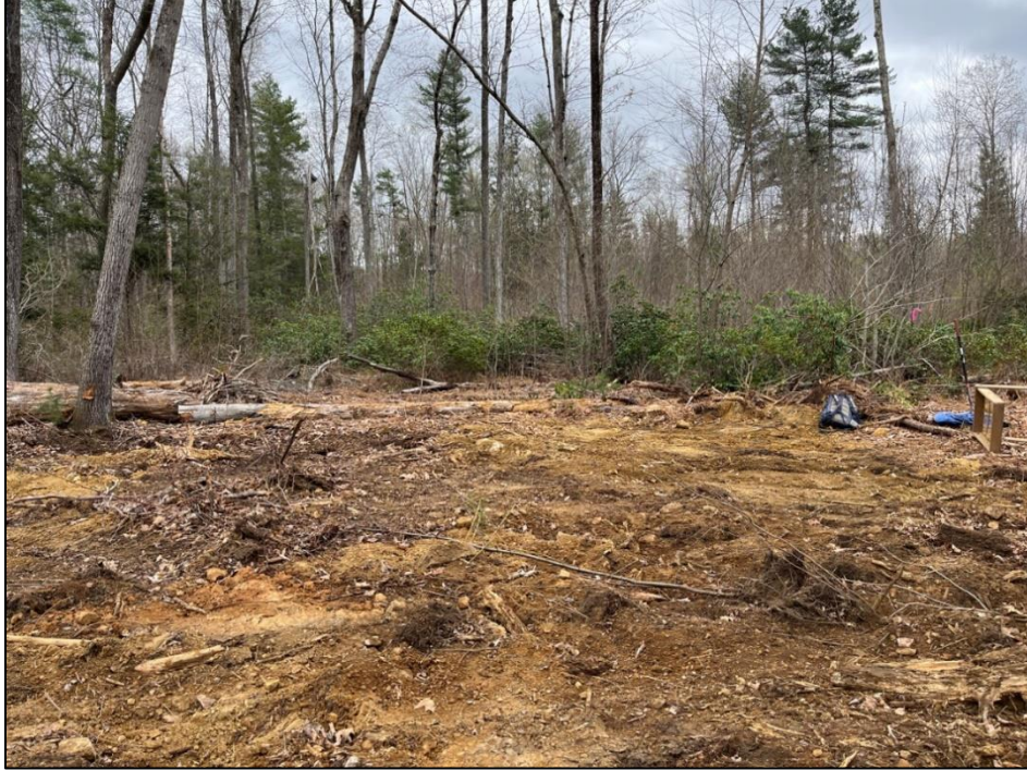
Photo 3. Overview of existing disturbance by bulldozer tracks and logging in the northern area of SA-1. Photo facing southwest.
