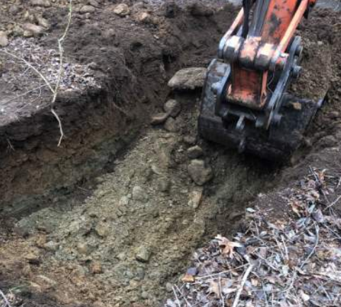
Bottom of test pit at 8.7 feet. Pictures showing soil strata at Test Pit 3
