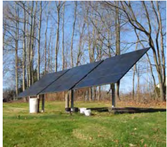
Residential solar panels
