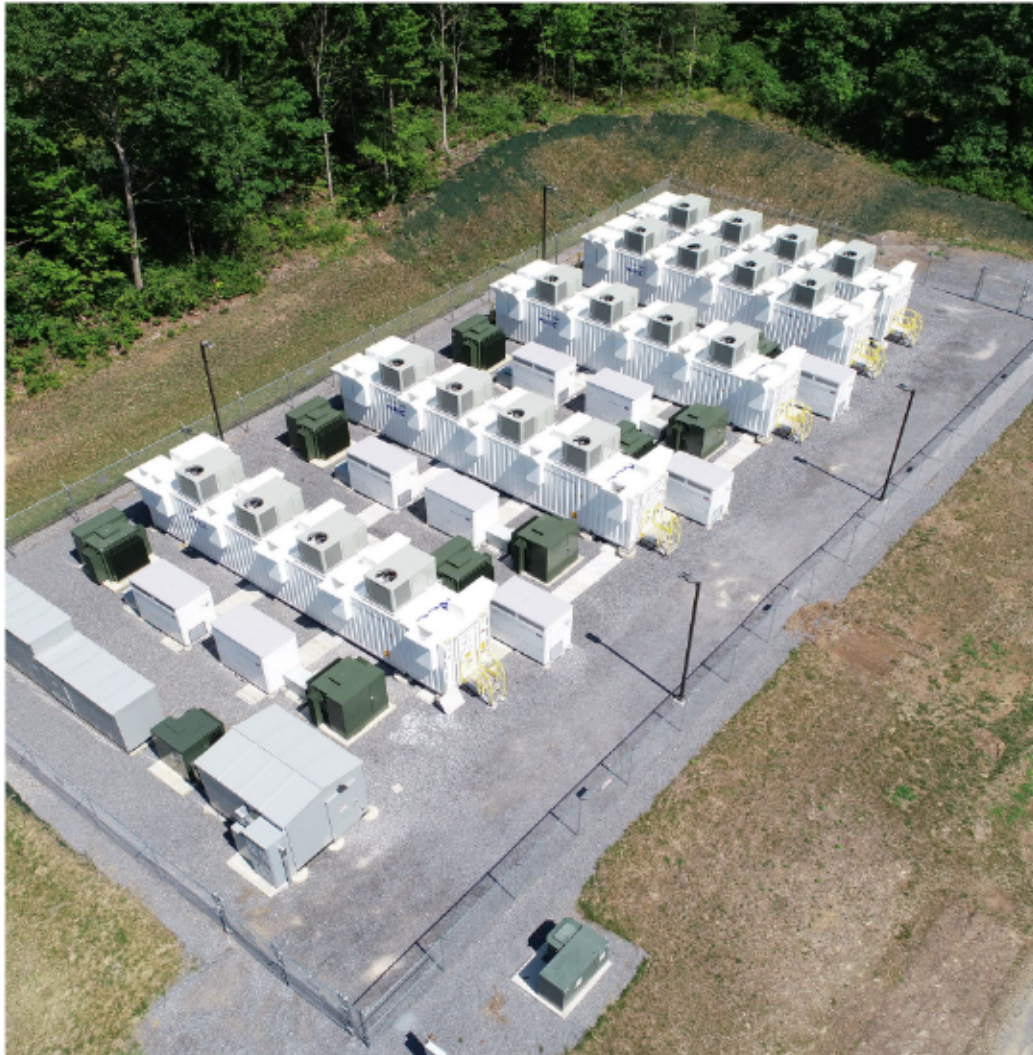
KCE's first operational project in New York, KCE NY 1, 20 MW/14.4 MWh BESS
