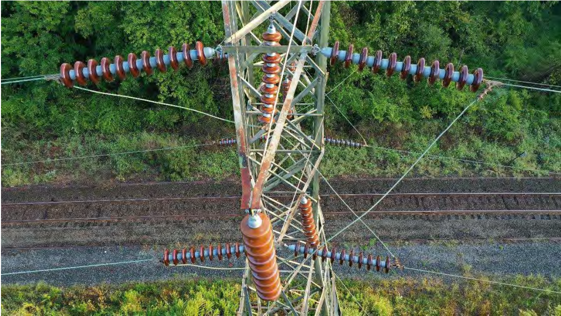
Structure 4644: rusting davit arm members
