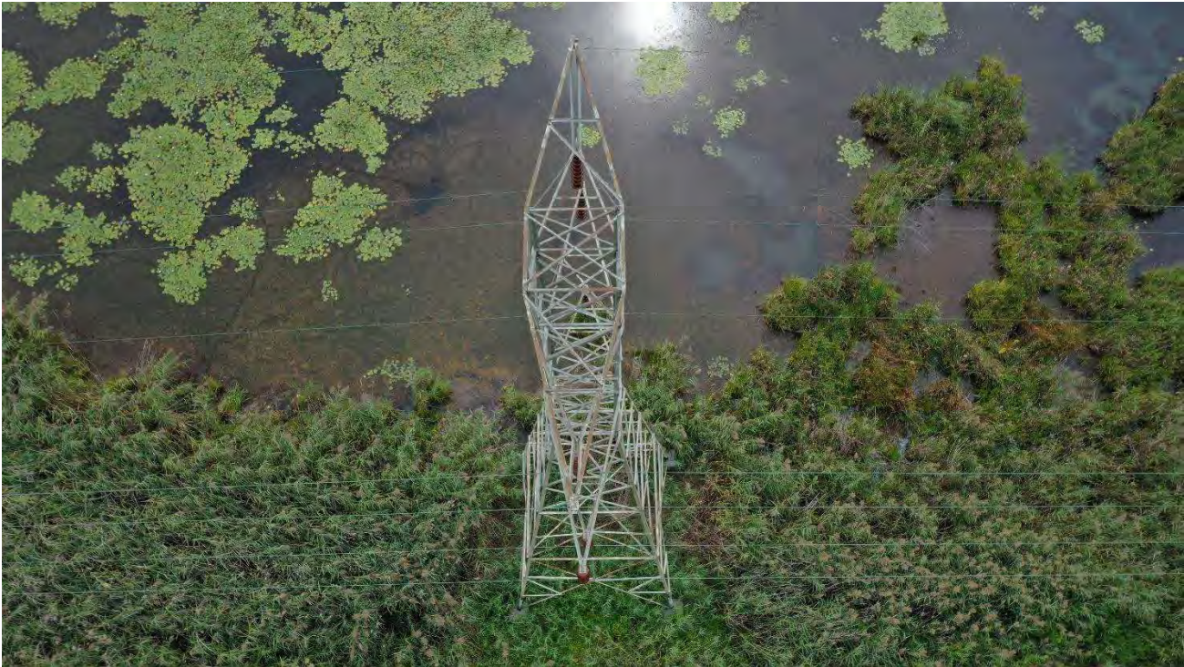
Structure 4642: rusting davit arm members
