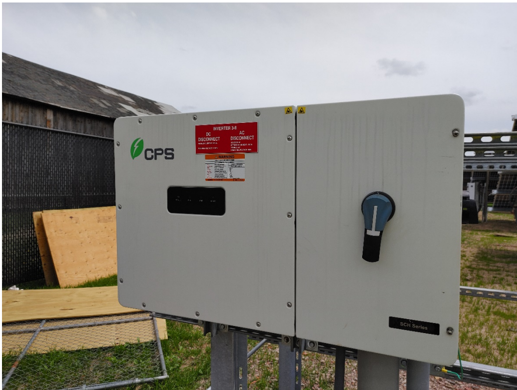
Tested Equipment – CPS Power Inverter – Sound measurement at 1 foot distance.
