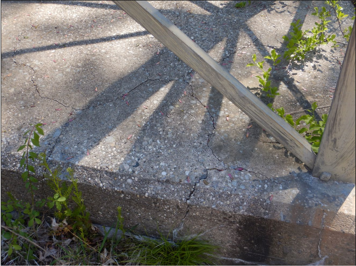
Structure 955 – Foundation Cracks
