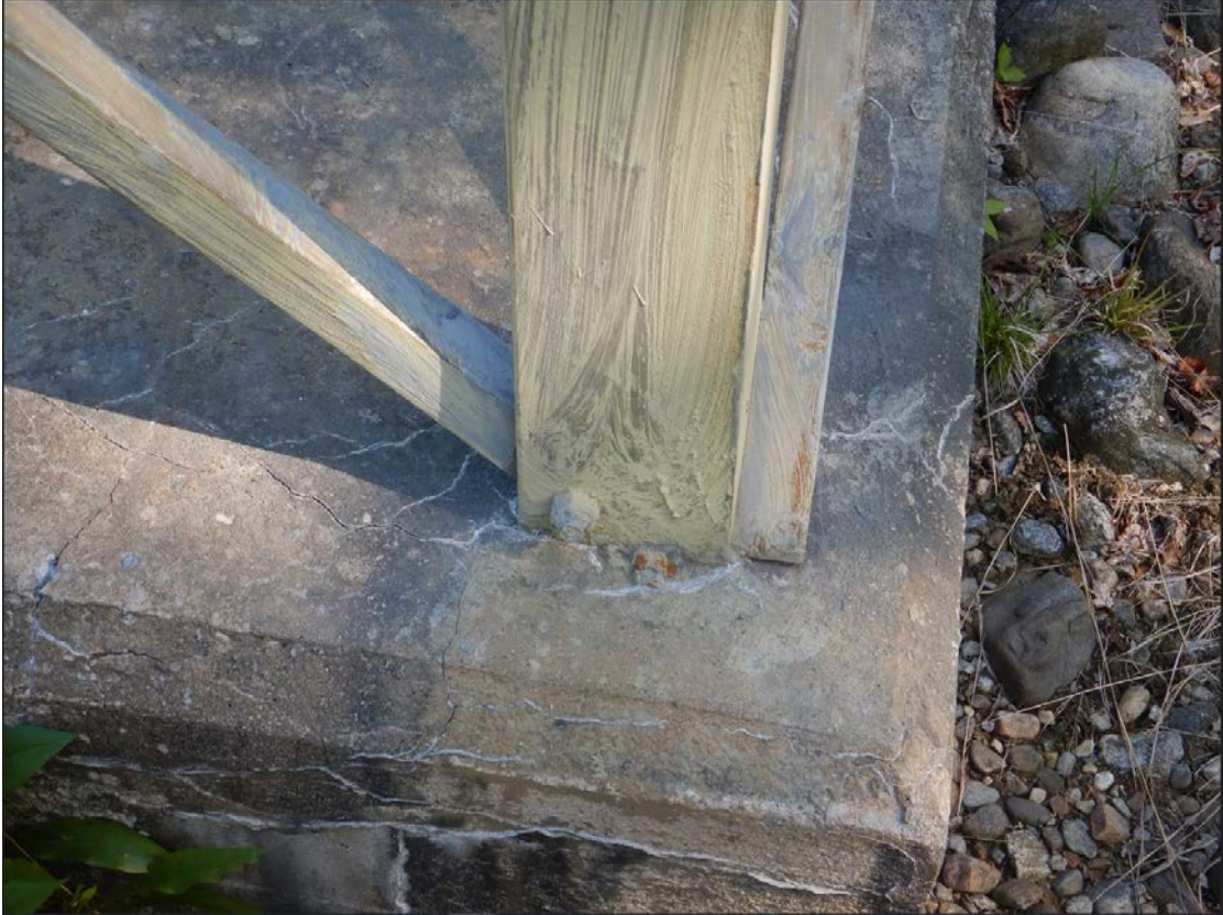
Structure 953 – Foundation Cracks
