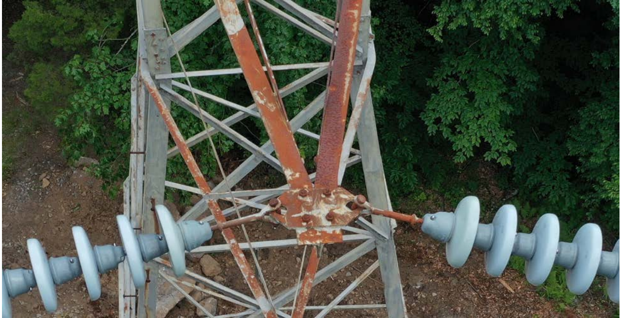
Structure 931 – Corrosion – pitting of tower arm members
