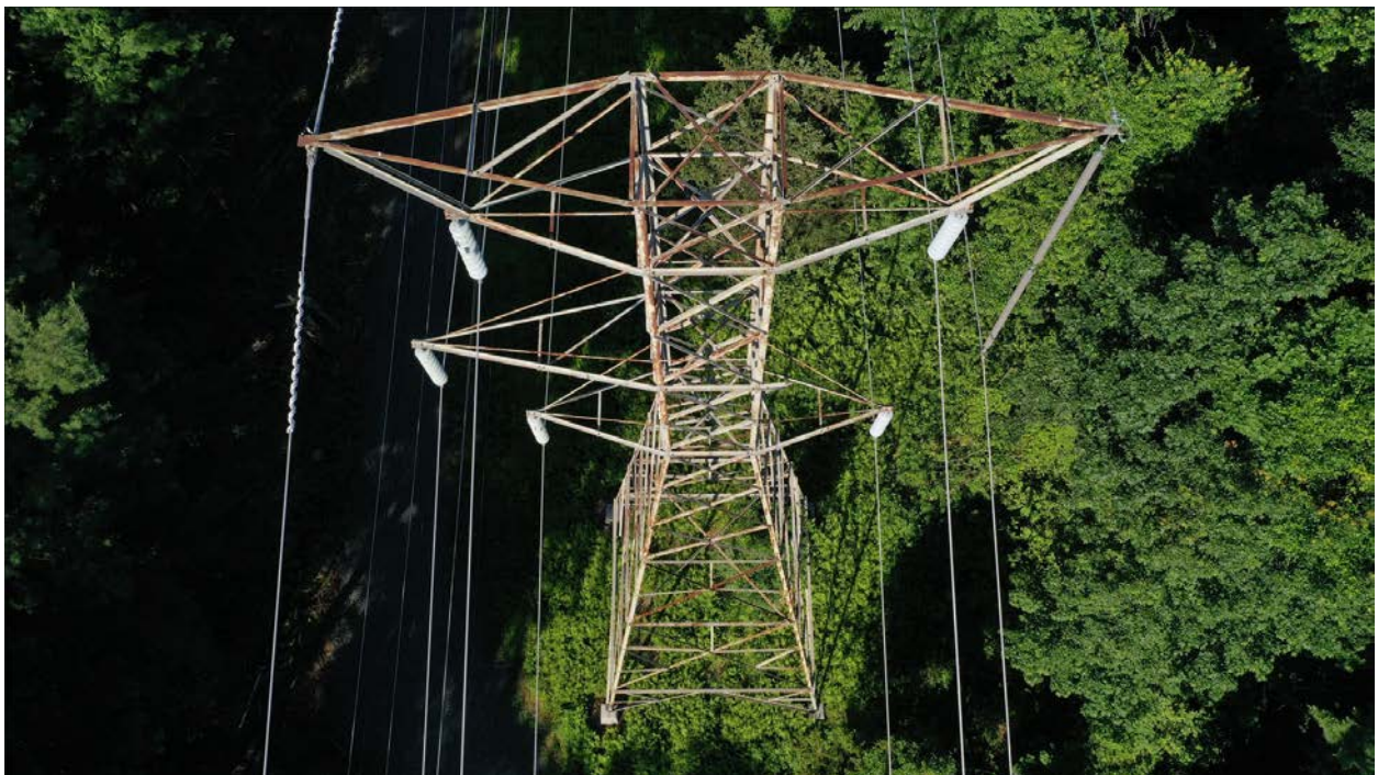
Structure 927 – Arm Damage due to Vegetation/Storm. (Arm damage has been repaired). Rust on tower members
