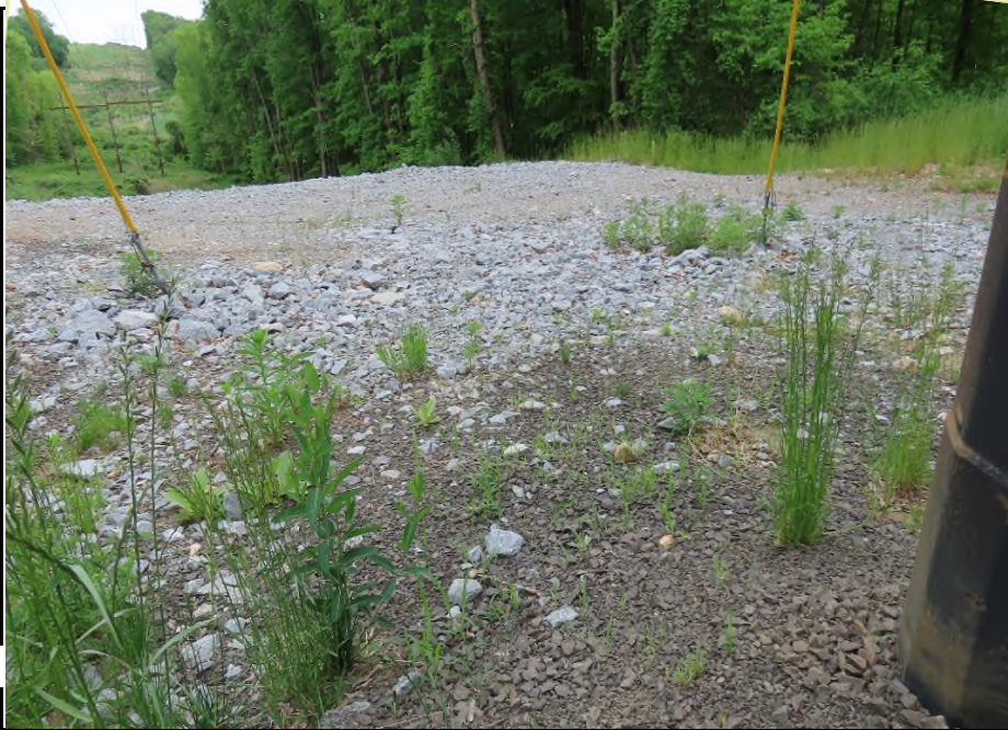
Photo 3-1. SW view downhill from sparse pad at Pole 7785 towards Pole 7784.
