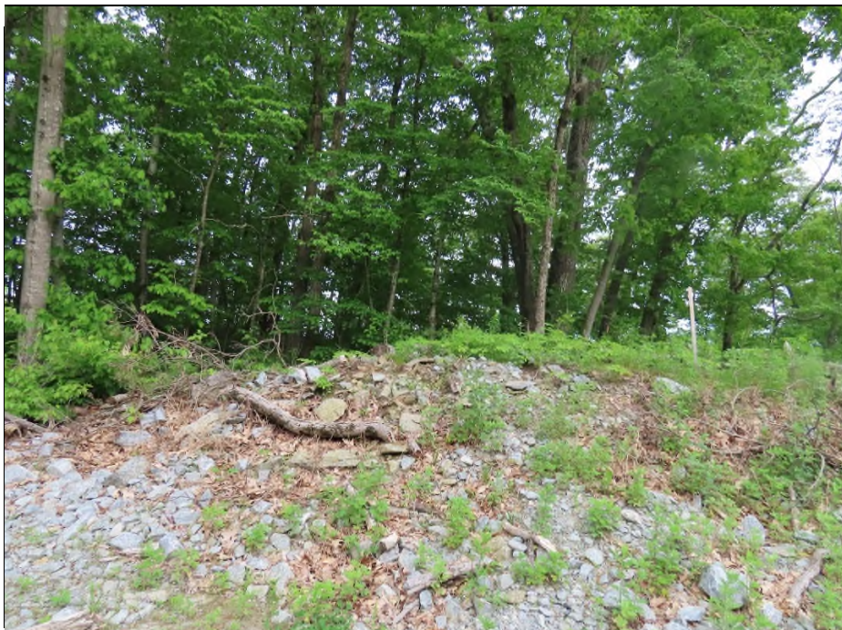
Photo 3-5. E. view. Cut & stone fill encroaches on Spaulding land, by Pole 7786.
