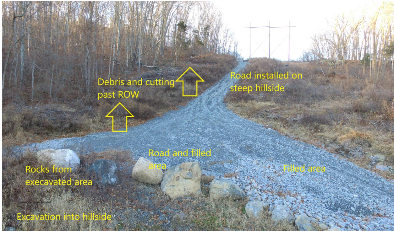
This is an image of the hillside and road from 7785 to 7786 which shows extensive erosion, suggesting poor design or construction, or both, creating a serious environmental problem:
