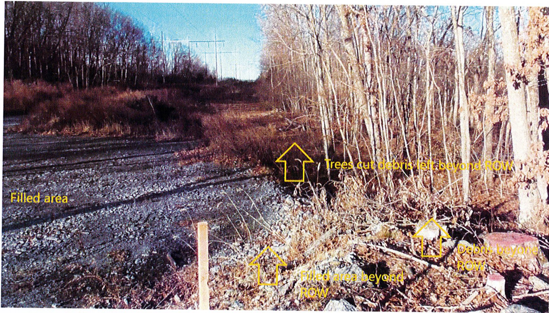
This photo depicts crushed rock fill deposited outside the easement and the debris left near site 7786.
