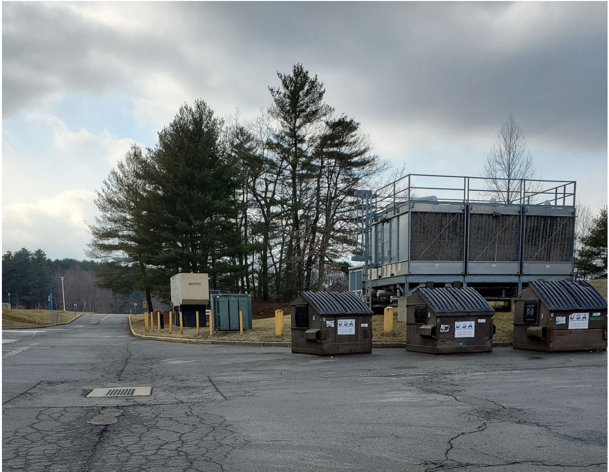
Looking west; Facility location beyond generator
