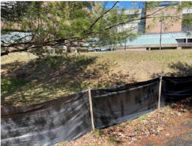
Image 1 – Front of Fuel Cell Install Area
