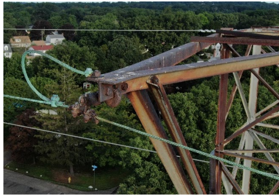
Structure 859 - rust on structure and hardware
