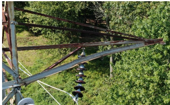
Structure. 897 - rust on structure and hardware and bent arm
