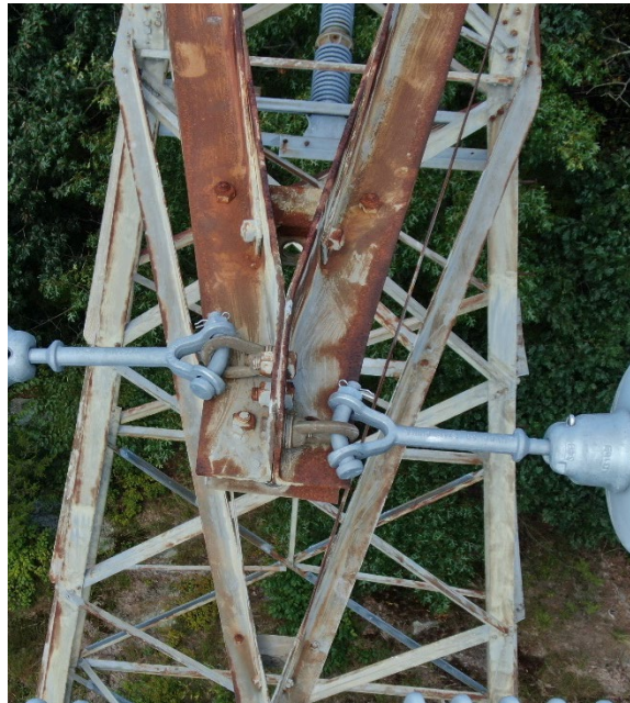
Structure 899 - rust on structure and hardware
