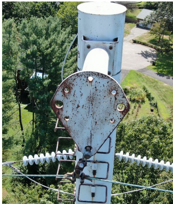
Structure. 872 - rust on structure and hardware
