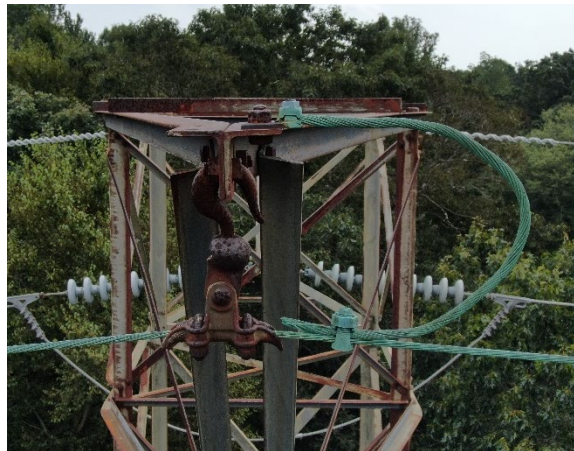
Structure 901 - rust on structure and hardware
