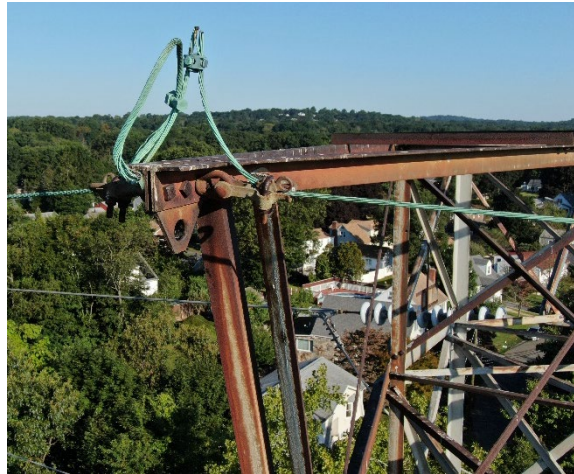
Structure. 860 - rust on structure and hardware
