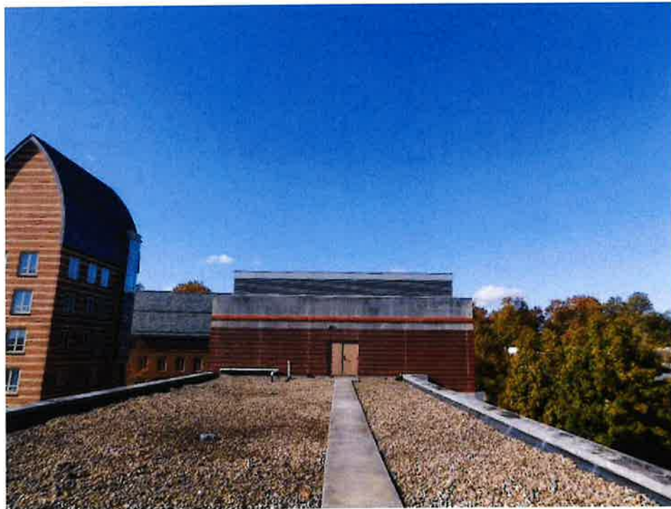
Photo 1: Sample photo illustrating the proposed location of the antenna enclosure (view from the East).
