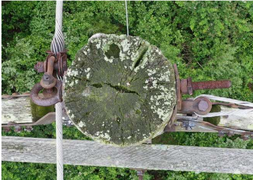
Structure 6311: Split top, Woodpecker Damage, cracks
