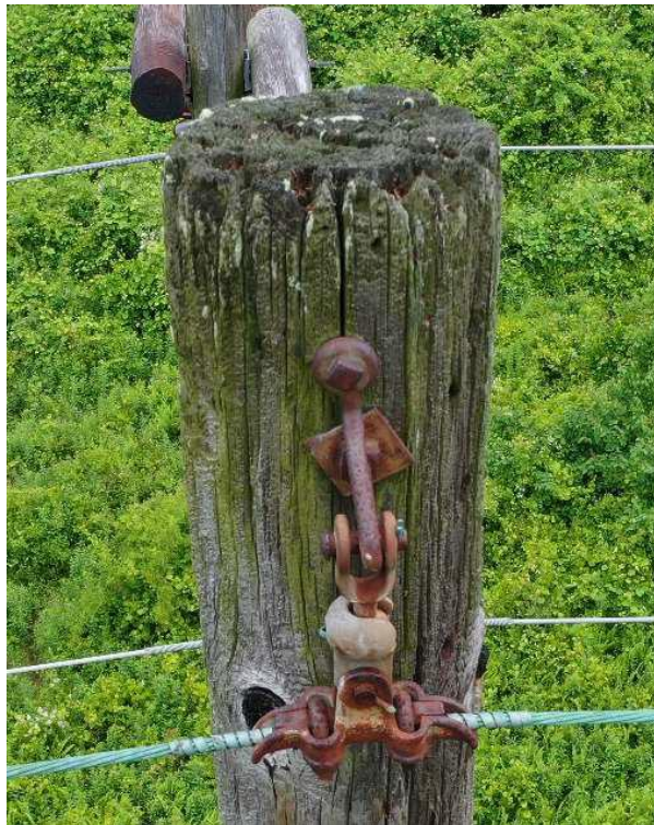
Structure 7617: Split tops, Woodpecker Damage, decay
