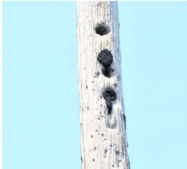
Structure 7656: Split tops, Woodpecker Damage, cracks in arm
