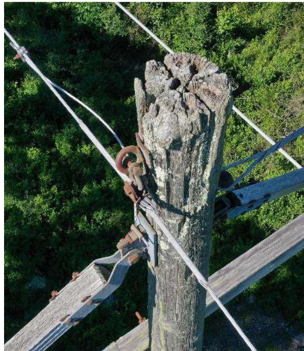
Structure 6358: Split top, cracks, decay
