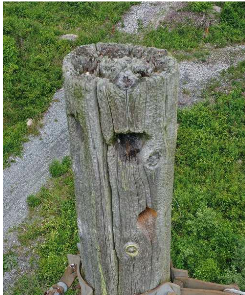
Structure 6320: Split top, Woodpecker Damage, cracks, decay
