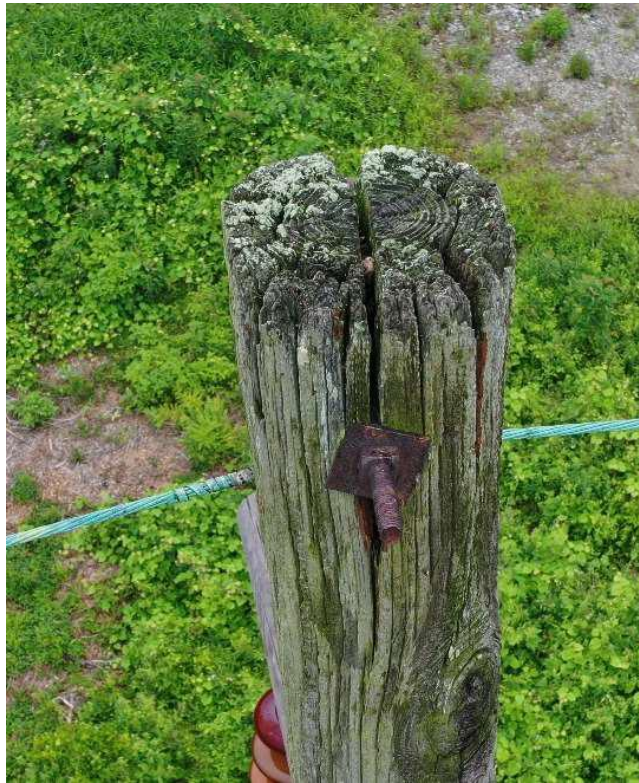
Structure 7619: Split tops, Woodpecker Damage, cracks, decay, cracks in arm
