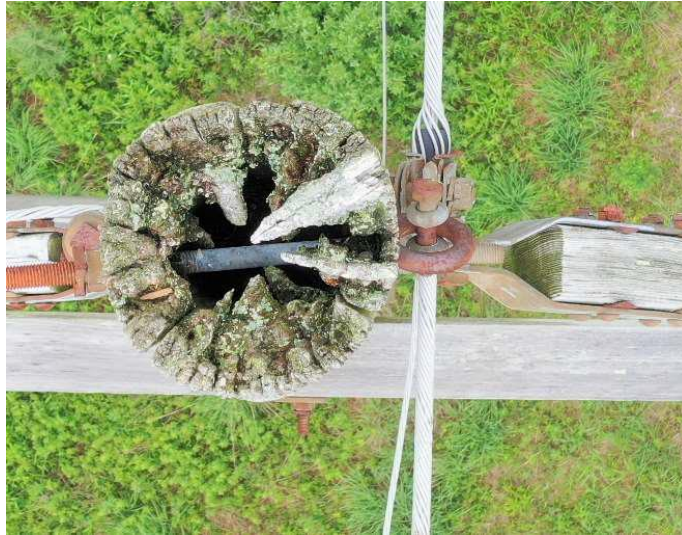
Structure 6318: Split top, Woodpecker Damage, cracks, decay
