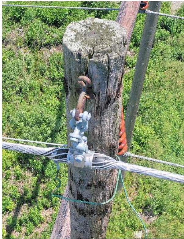
Structure 7659: Split tops, cracks, decay
