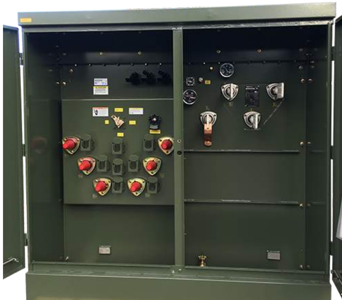
Fig 2. Three Phase Maddox Padmount Transformer
