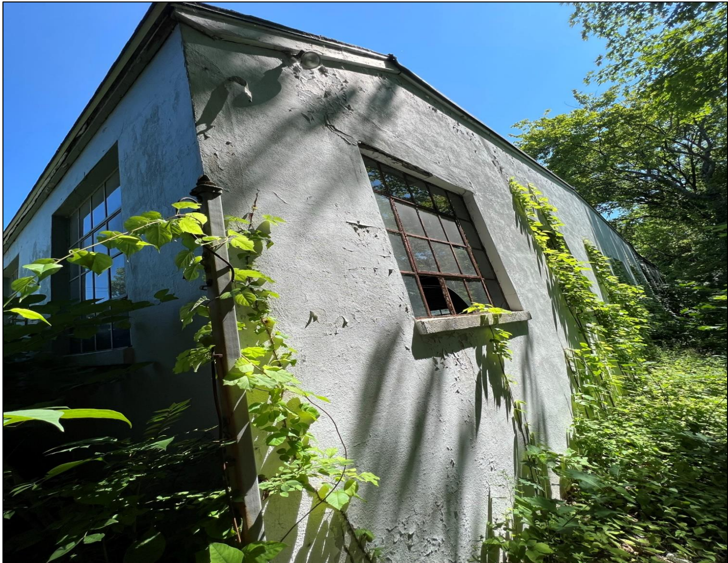
Photo 8. Detail photo of rear wall of existing structure in project area, looking northeast.
