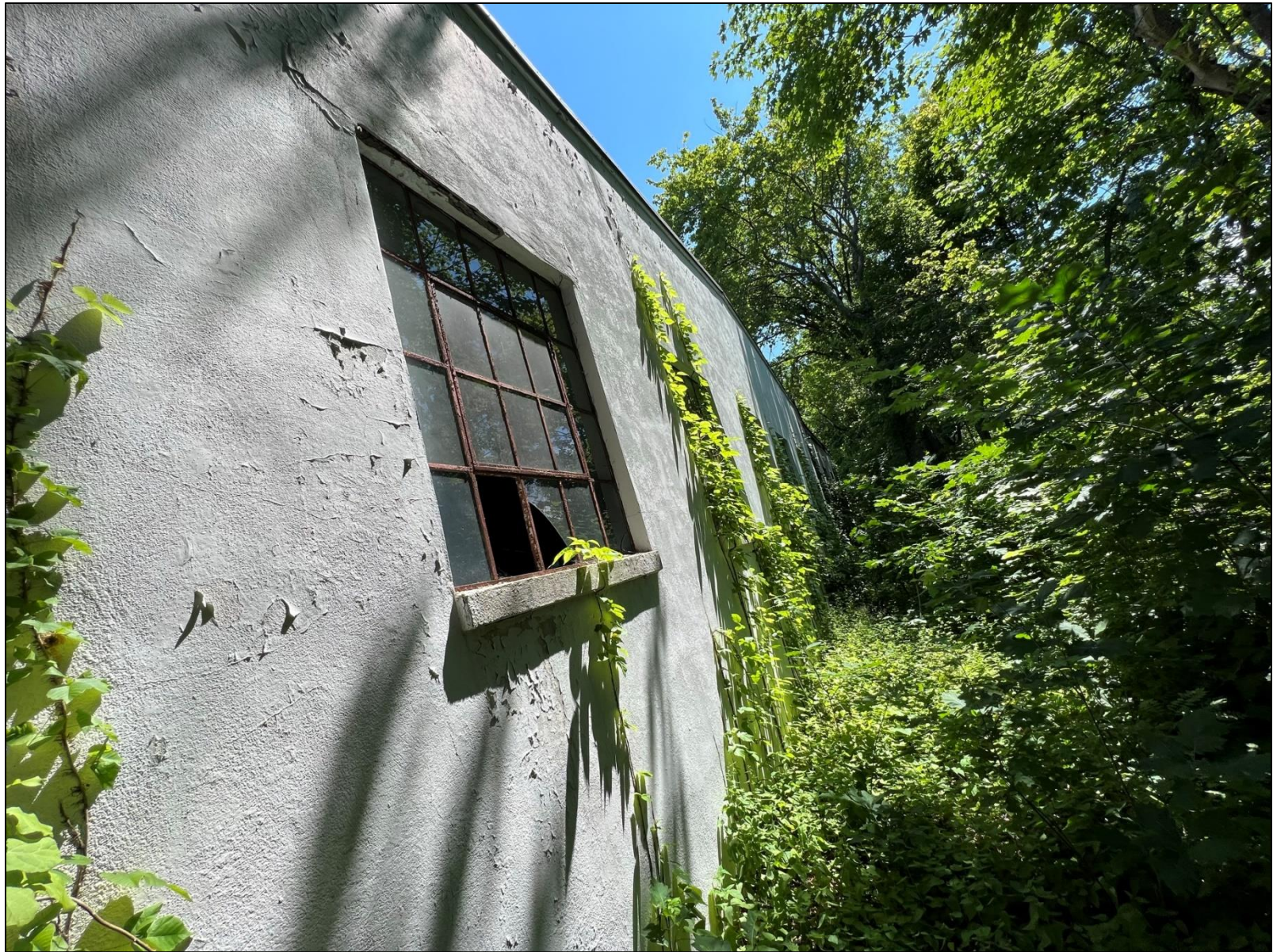
Photo 9. Detail photo of rear wall of existing structure in project area, looking east.
