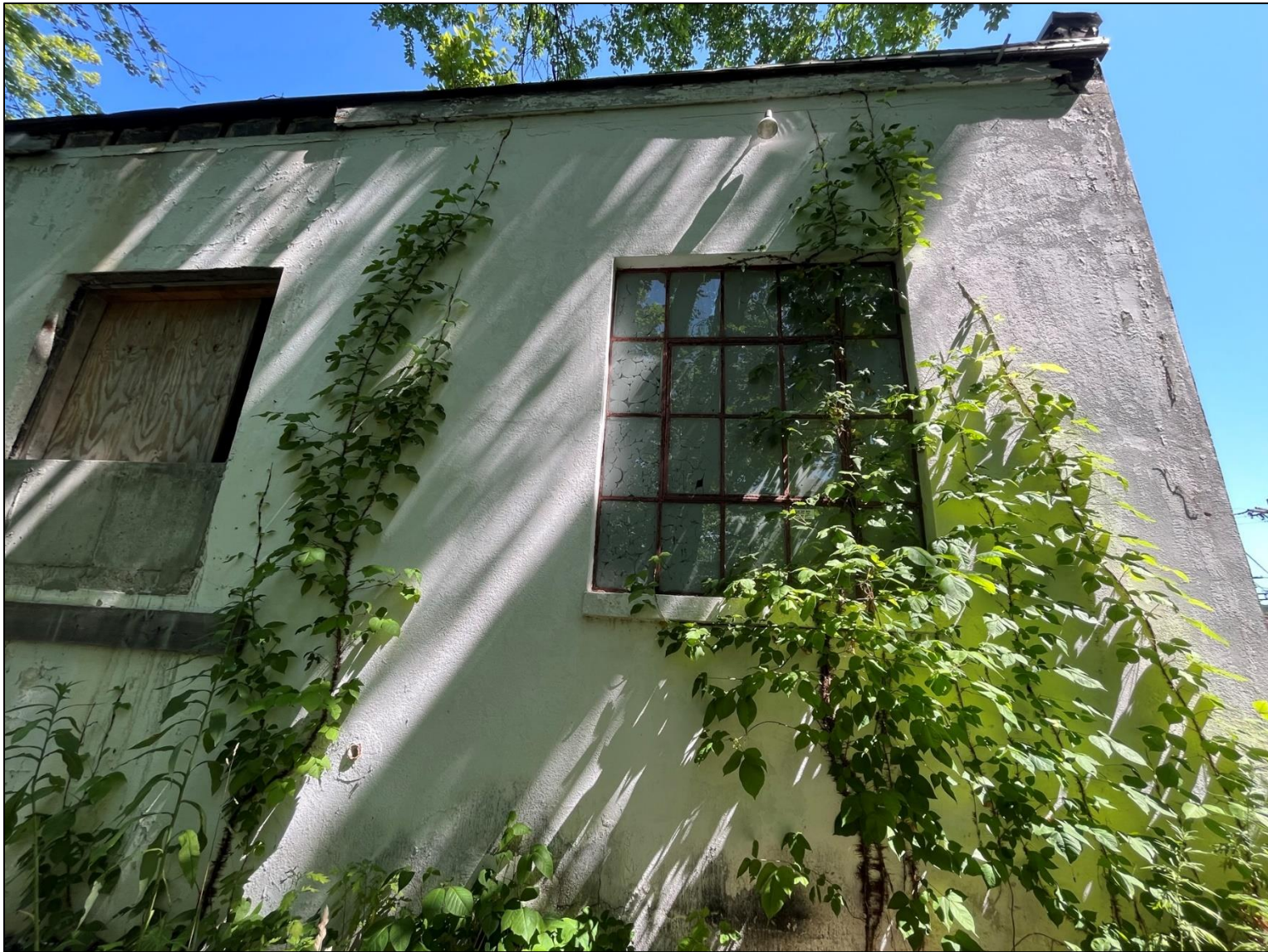
Photo 6. Detail photo of rear wall of existing structure in project area, looking northwest.
