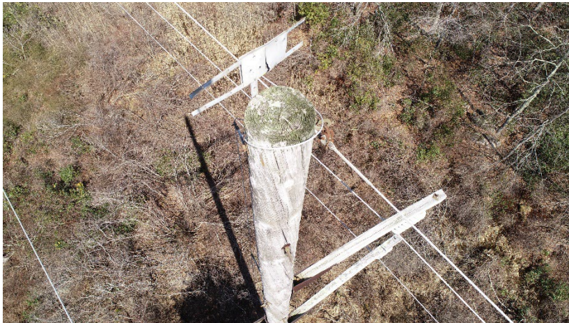
Structure 125: Pole top rot
