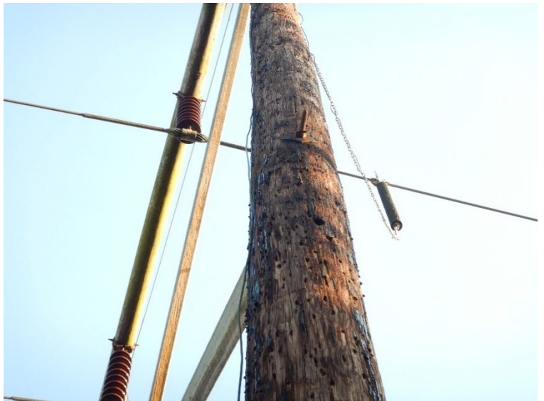
Structure 8388: Woodpecker Damage and rotted pole
