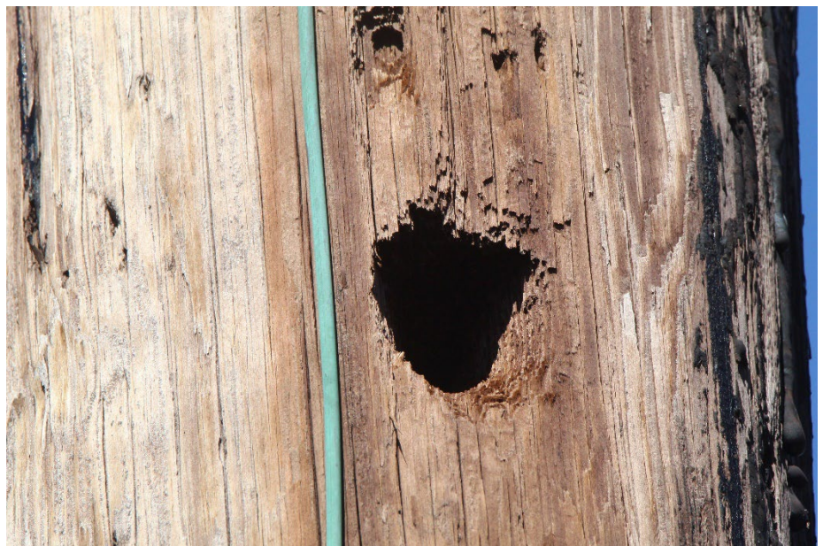
Structure 8374: Hollow Pole and severe woodpecker damage
