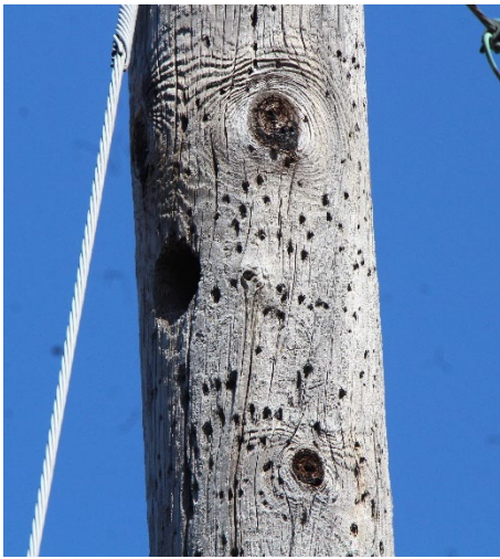
Structure 8387: Woodpecker Damage and rotted pole
