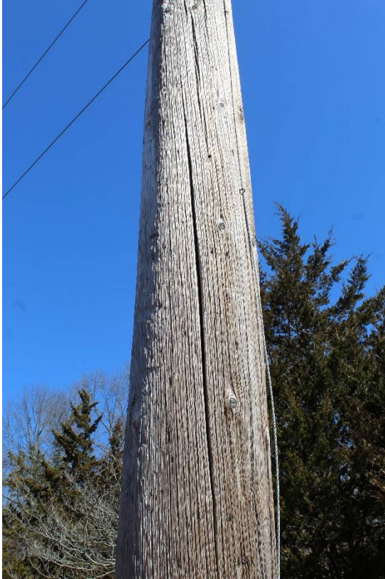
Structure 122: Pole cracks
