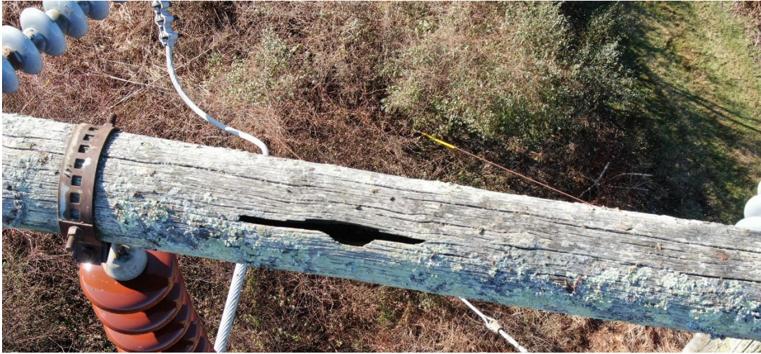
Structure 8430: Rotted arms and cracks
