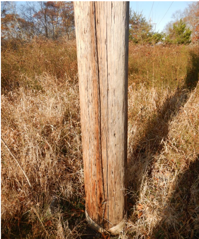
Structure 8389: Cracks and rot
