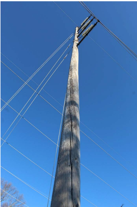
Structure 115: Severe Cracks
