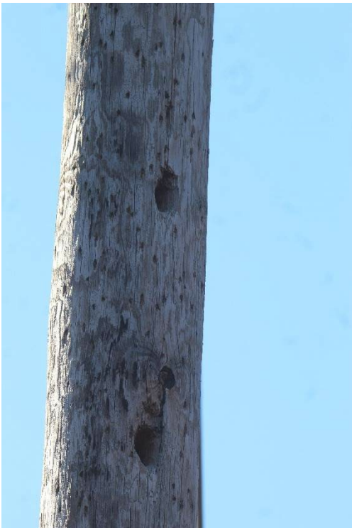
Structure 8370: Woodpecker Damage
