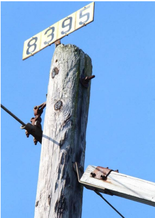
Structure 8395: Woodpecker Damage and rotted pole
