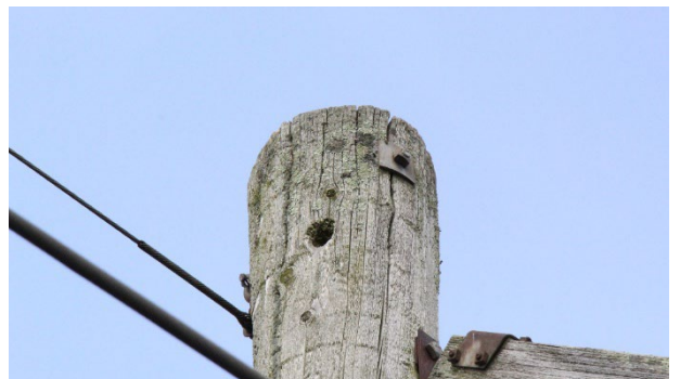
Structure 8431: Rotted pole tops and Woodpecker damage
