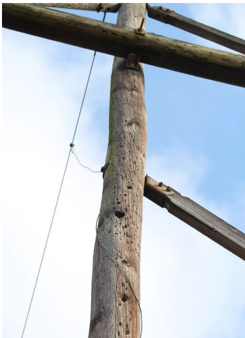
Structure 8420: Woodpecker damage
