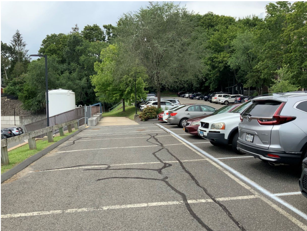
Looking west from within Energy Server location toward associated equipment area
