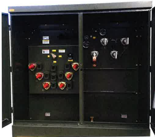
Fig 2. Three Phase Maddox Padmount Transformer
