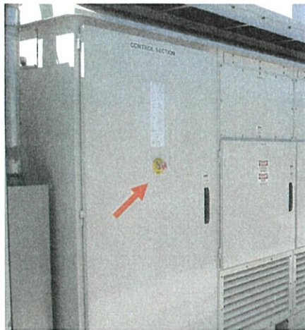
Electrical Balance of Plant
