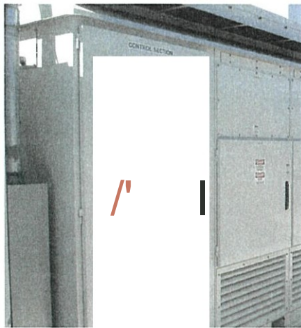
Electrical Balance of Plant
