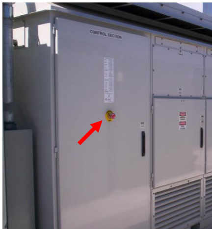
Electrical Balance of Plant
