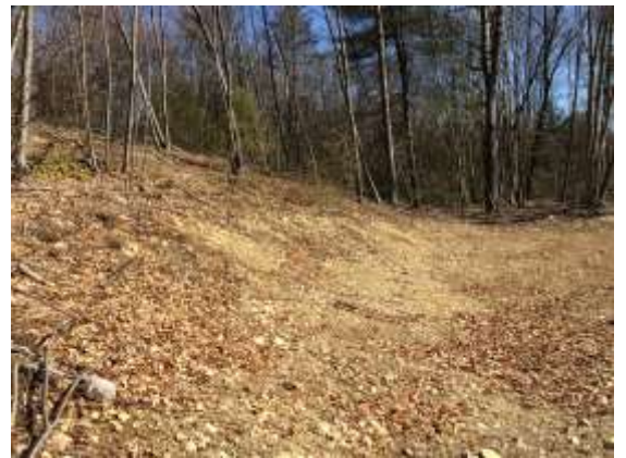
Figure 5. Sparsely vegetated recently cleared and excavated area at the southwest corner of the Project Area.
