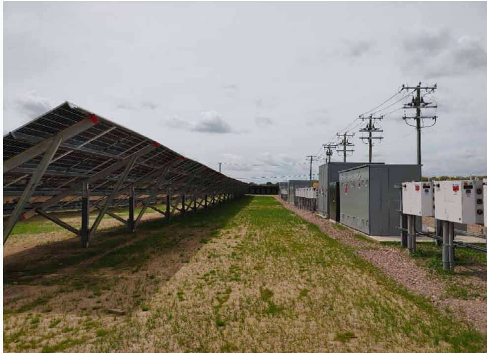
Figure 2, a. Solar panels, power inverters, electric switchgear and transformers, and overhead transmission lines. Viewing west.
