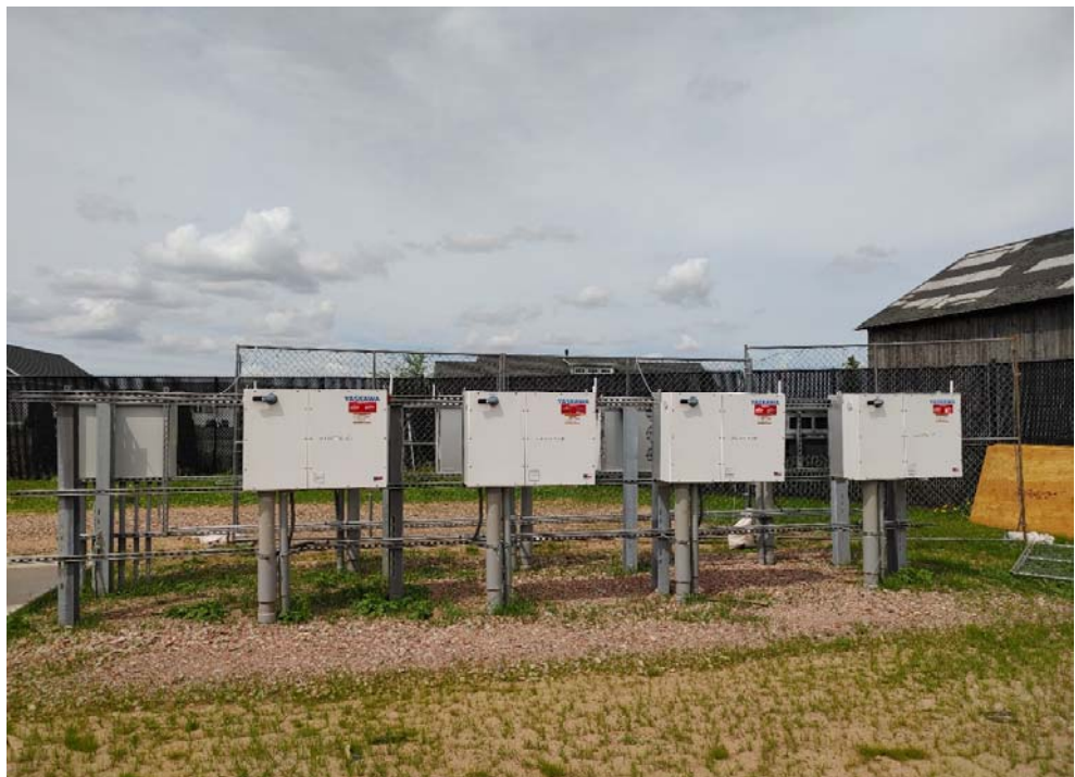
Figure 2, b. Solar power inverters. Viewing north.
