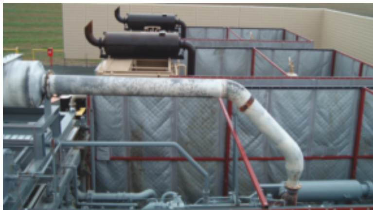
BBC-EXT-R-2" Sound Curtains enclose pumps and compressors.
