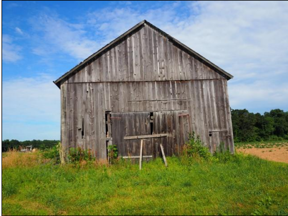
Figure 37. Frontal view of Tobacco Shed No.3 facing east toward Barber Hill Road.
