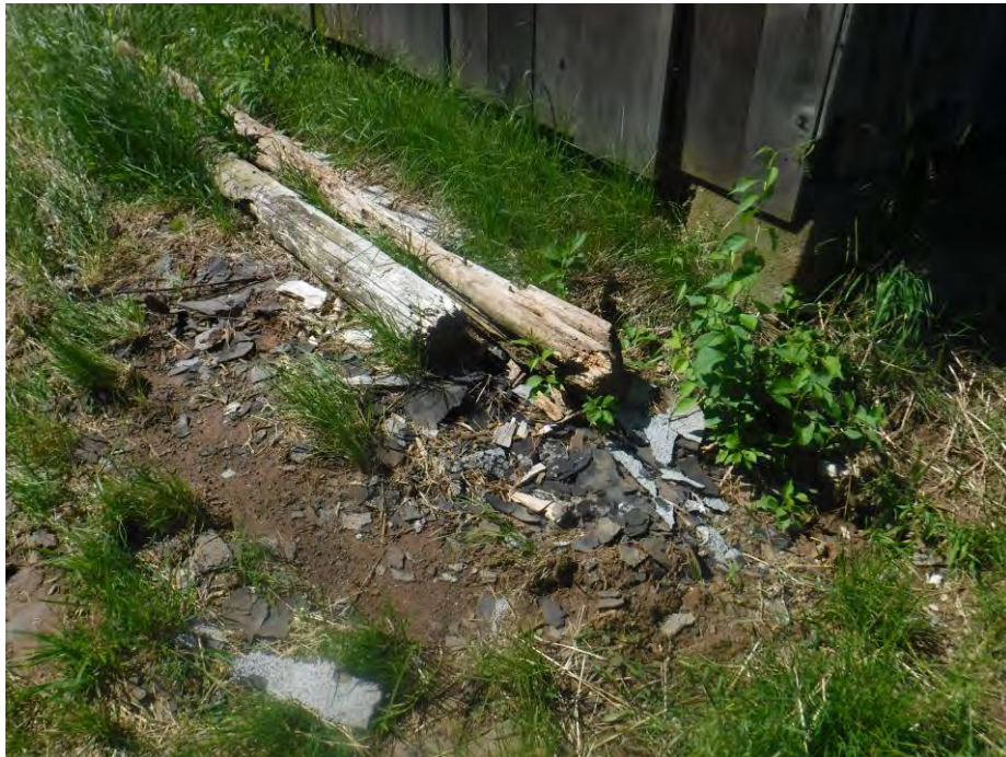
Photograph 6: 038-68-030 - Wapping Road, asphalt shingle material outside barns
