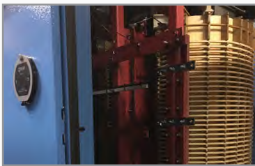
Infrared viewing window & custom enclosure finish
