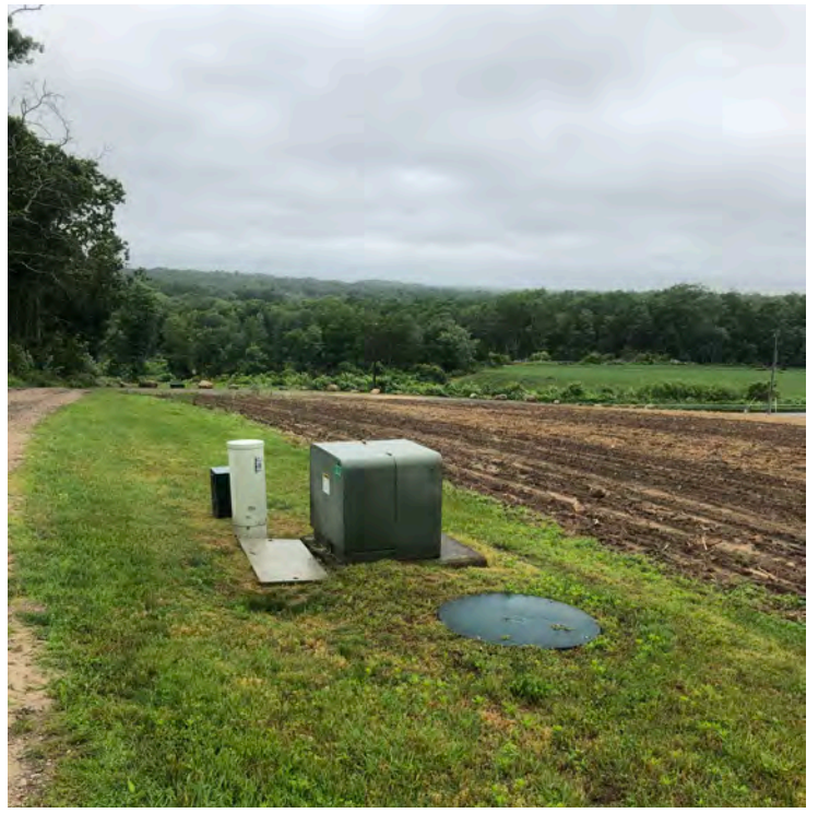
Parcel 119-6313, utility vaults and transformer.
