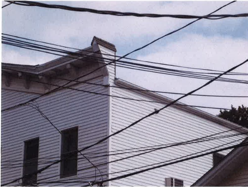
Photo 1: Sample photo illustrating the proposed location of the new antenna (secured on the back side of the parapet).
