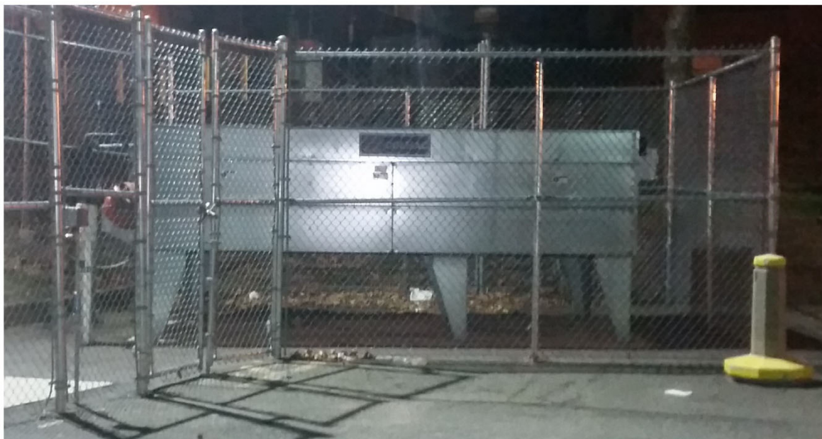
Figure 2. Doosan Fuel Cell Cooling Module at the Mount Sinai Hospital Site in Hartford CT
