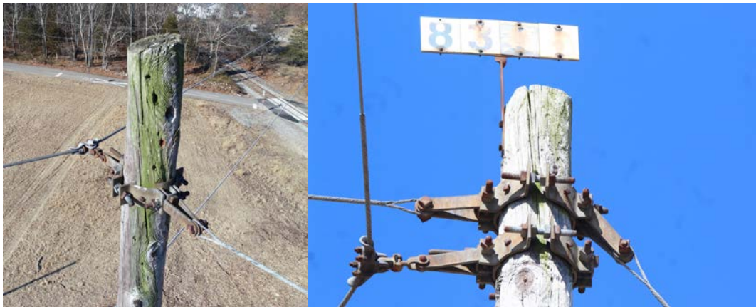
Str. # 8345: Split pole tops.
