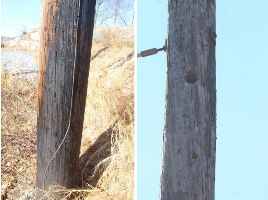
Str. # 8344: Wood pecker damage, burnt at base.
