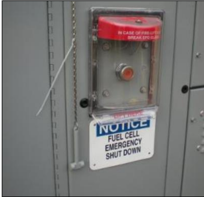
Figure 1: Emergency Power Off Button
