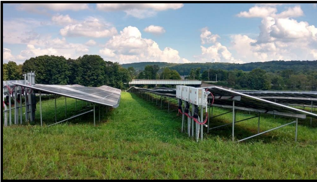
Picture 1 - Typical ground cover around solar arrays (Windham Solar 2019)
