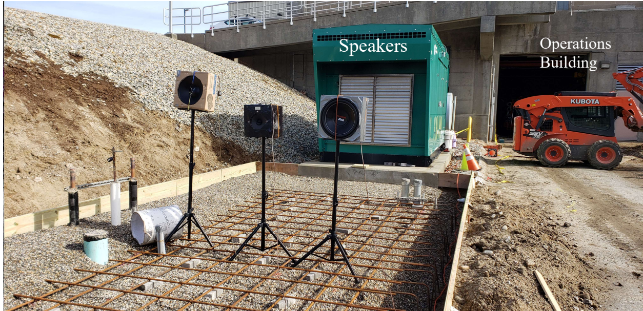
Figure 2. Doosan Fuel Cell Location at the Montville VFS, LLC Site
