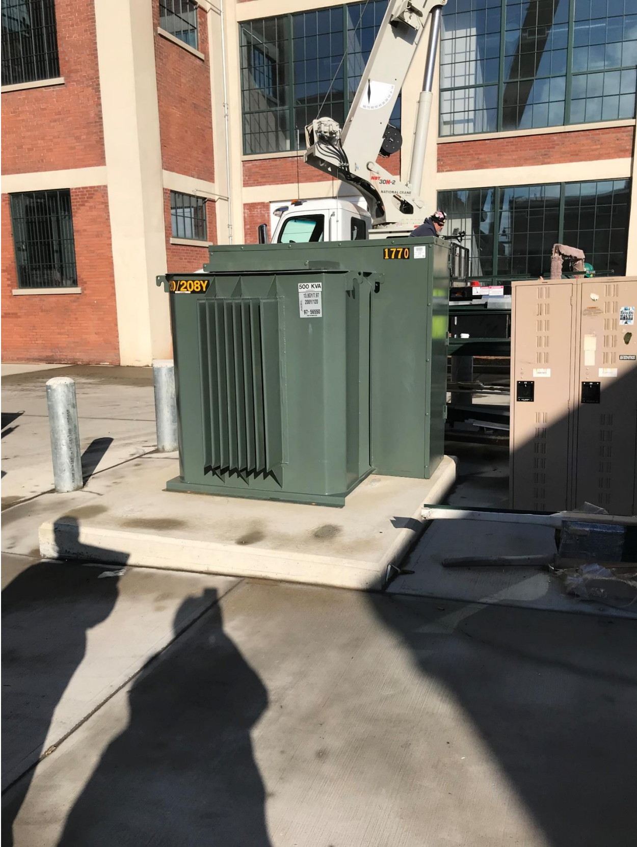
Fuel Cell Area in Courtyard of Cherry St Lofts Attachment #2
