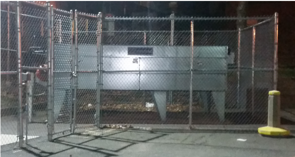
Figure 2. Doosan Fuel Cell Cooling Module at the Mount Sinai Hospital Site in Hartford CT
