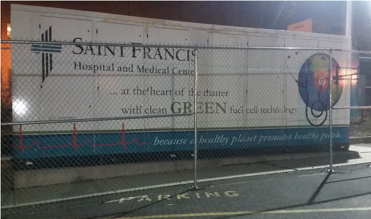
Figure 1. Doosan Fuel Cell Power Module at the Mount Sinai Hospital Site in Hartford CT
