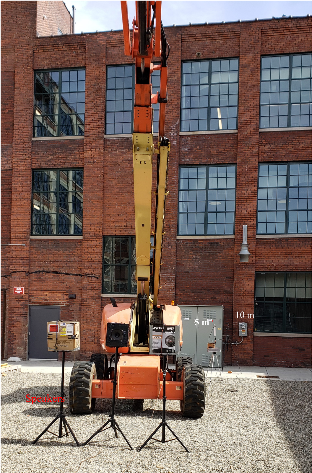
Figure 3. Position B Fuel Module Location at the Bridgeport Cherry Street Lofts Site
