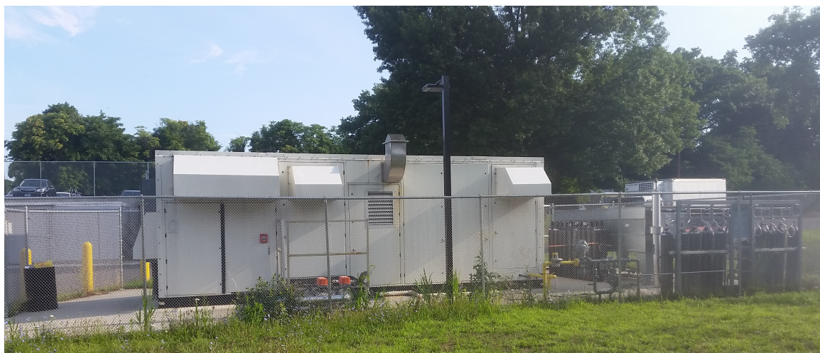
Figure 6. New Britain Power Module Showing the Fan Side of the Unit
