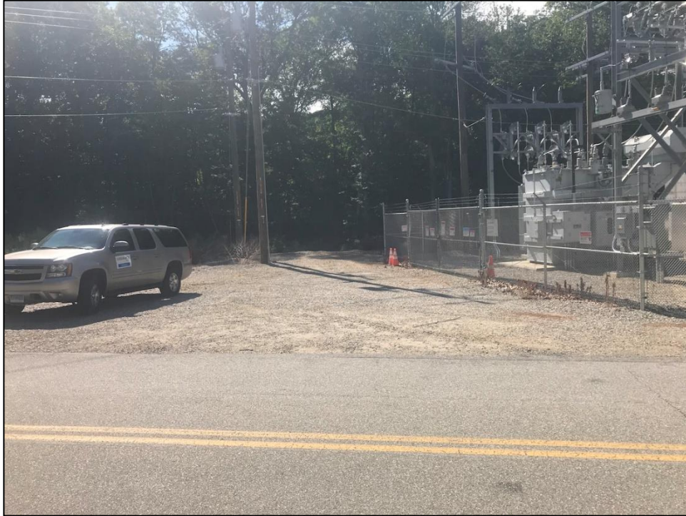
Figure 14. Overview of the northern portion of the project parcel and the existing Eversource Energy substation.
