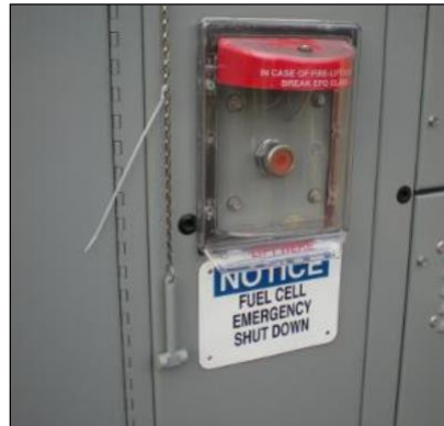
Emergency Power Off Button
