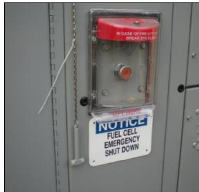
Emergency Power Off Button
