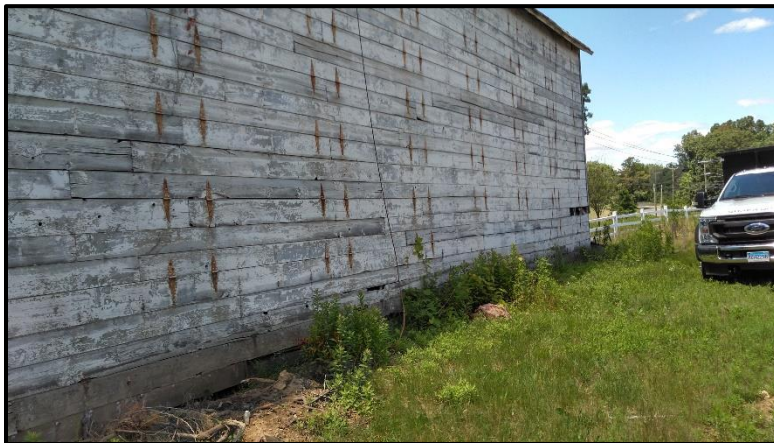
(Missing board #1 before [corner of barn])
