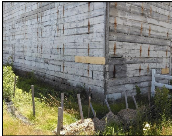
(Missing board #1 after)
