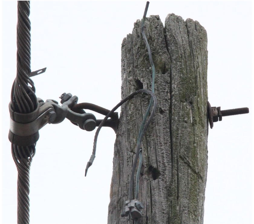
Str. # 52. Split pole tops, cracks woodpecker damage, damage at base of pole.
