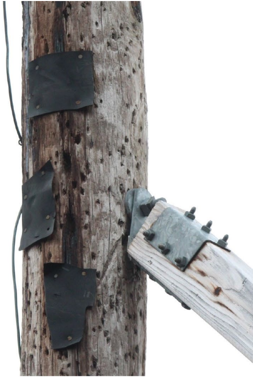
Str. # 50. Split pole tops, cracks, woodpecker damage and inverted fiber.
