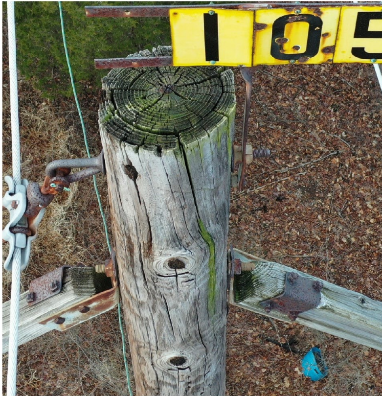
Str. # 105. Split pole tops, shell rot, woodpecker damage and wood decay.
