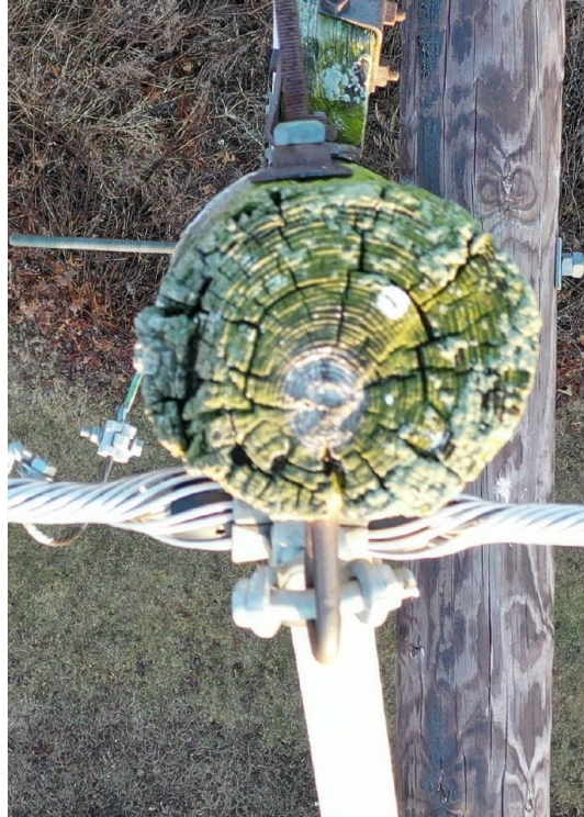
Str. # 111. Split pole tops, shell rot, woodpecker damage and cracks.
