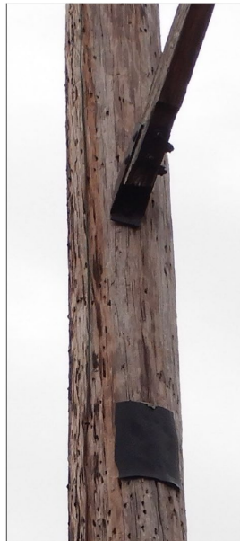
Str. # 55. Split pole tops, cracks, woodpecker damage, disconnected guy wire and 1 broken bell
